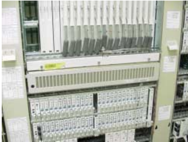
Figure 13. Temporary Location of DS3 Coaxial Cables
