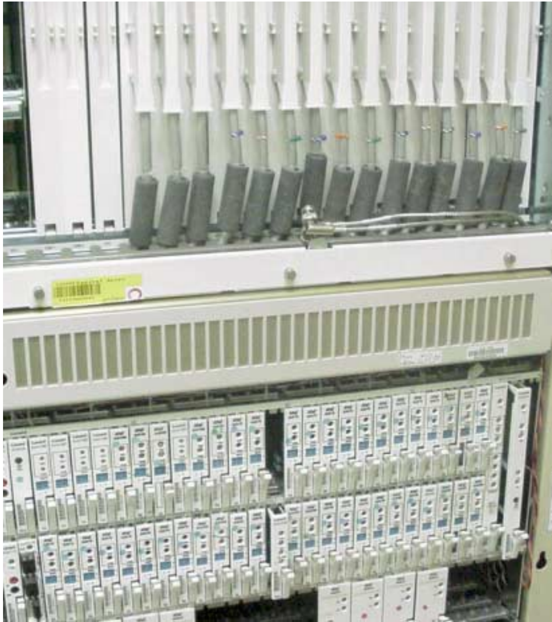
Figure 7. General View of Fan Orientation and DS0/DS3 Wiring
