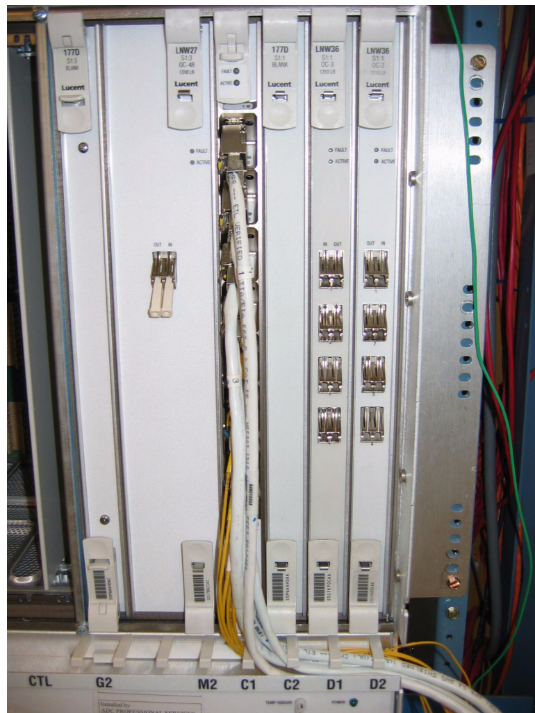
Figure 1-19 Ethernet cable routing to faceplate SFP modules
