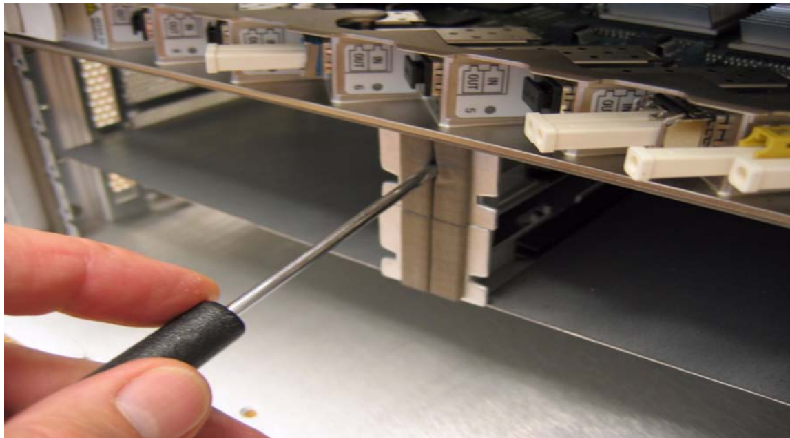
Figure 2-4 Center divider with circuit packs installed.
